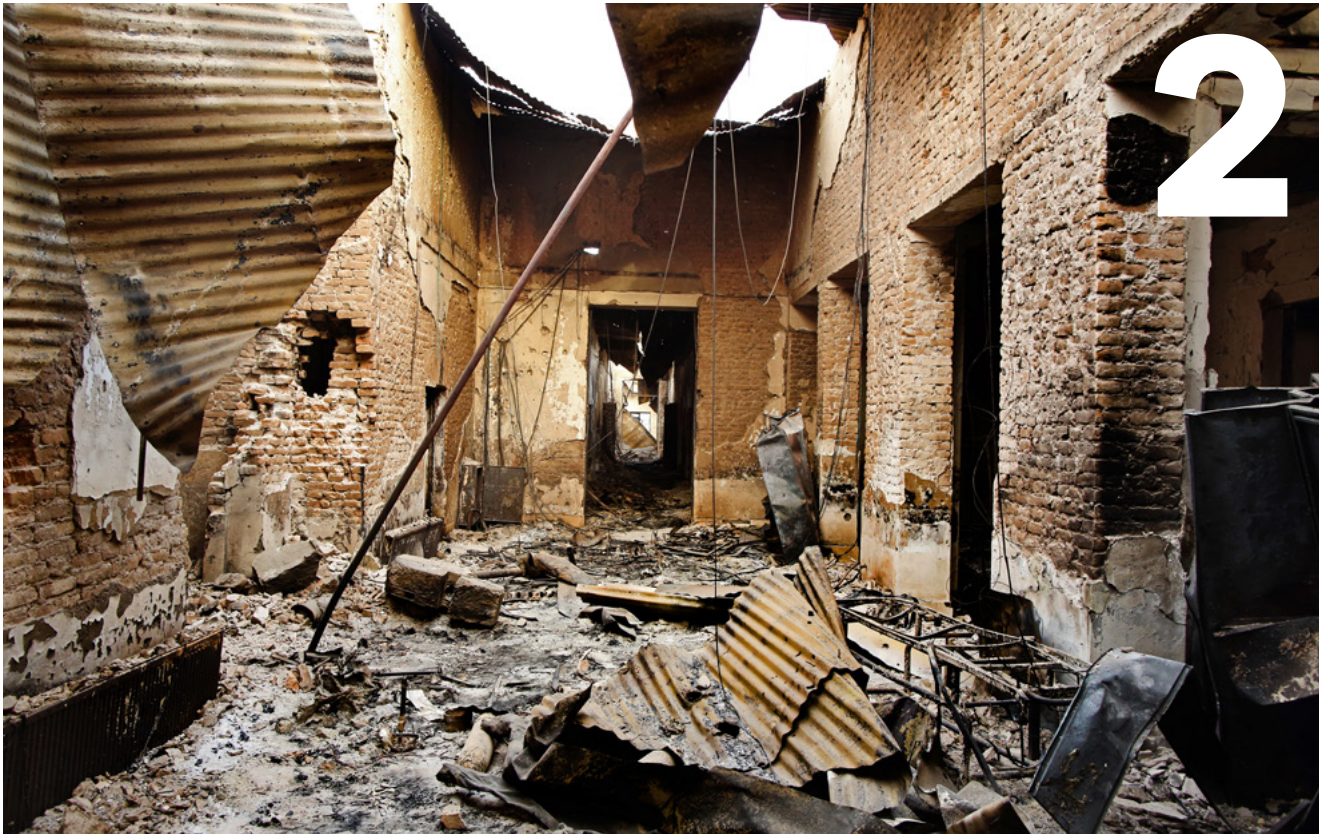
↑ Iron roofing and rubble litter a corridor in the MSF Kunduz Trauma Centre as the facility lies destroyed following the 03 October aerial attack which killed 42 people including 14 MSF staff members and patients in northern Afghanistan. October 2015. Photo: Andrew Quilty.
