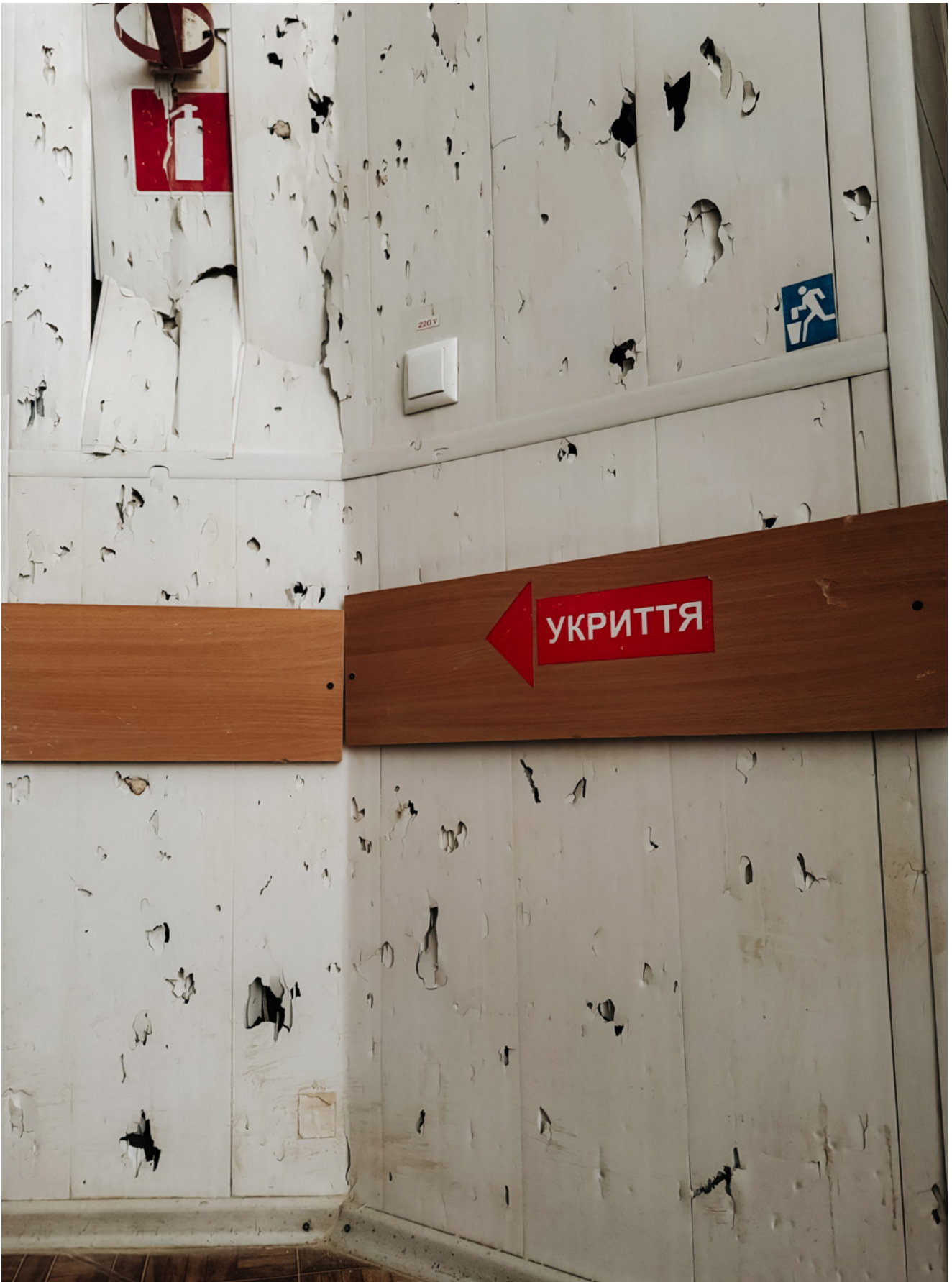
↑ First of July, Russian forces shelled a hospital in Kherson. A few days later, when we arrived, medical personnel had already begun to clean and repair the damaged parts of the building. But the consequences of the attack were brutal and clearly visible. We found glass from the broken window in a pot nearby. What was striking for me is that the hospital continues to operate, providing help for patients. Ukraine, July 2025. Photo: Yuliia Trofimova/MSF.
