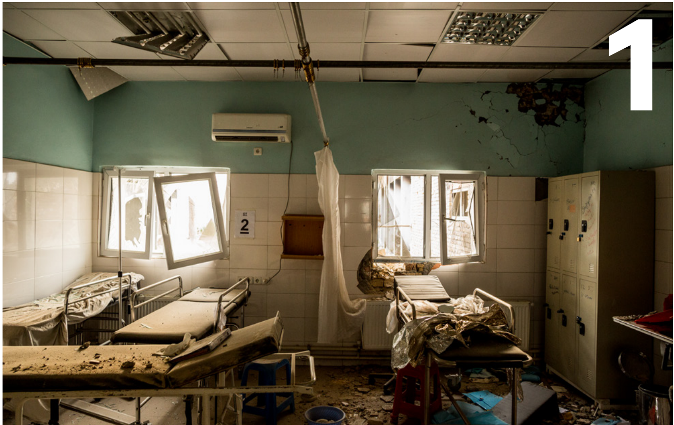
↑ Burnt-out corridors, collapsed roofs, twisted metal and ash, is all that remains of many building at the MSF Trauma Centre in Kunduz, northern Afghanistan, following the 03 October US airstrike on the facility which killed 42 people including 14 MSF staff members and patients. Afghanistan, 10 October, 2015. Photo: Andrew Quilty.
